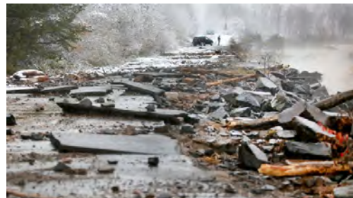
Here's can happen to recreational infrastructure when we do not keep changing water levels in mind (Duluth News Tribune)
