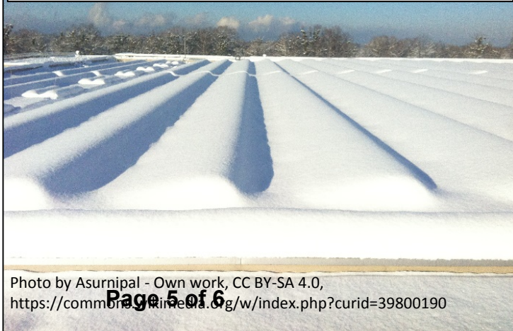
“Buried” - commercial roof-top solar
