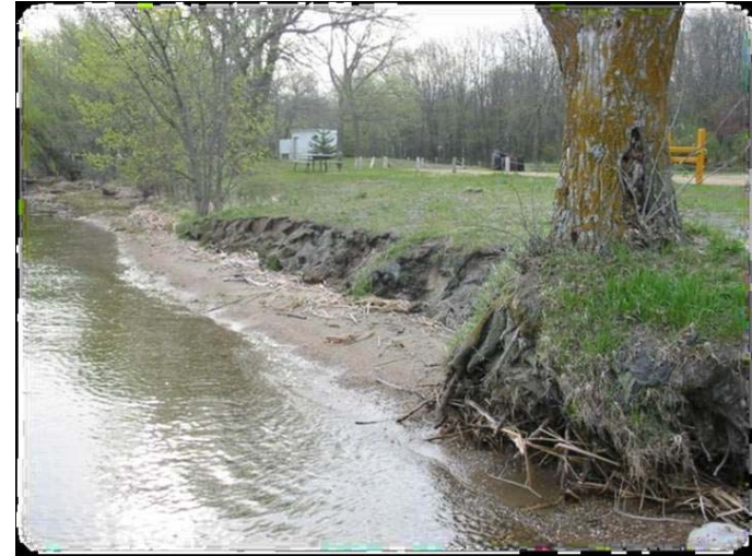
Example of Degraded Stream Bank
