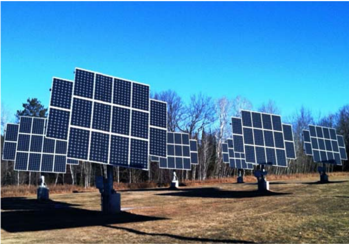
Figure 1: This photovoltaic system consists of 9 dual tracking arrays and is located at the Audubon Center of the Northwoods in Sandstone, MN.
