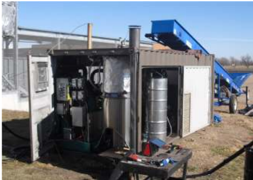
“PowerTainer” installed at UM Morris
