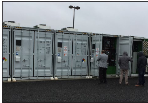
exterior of flow batteries
