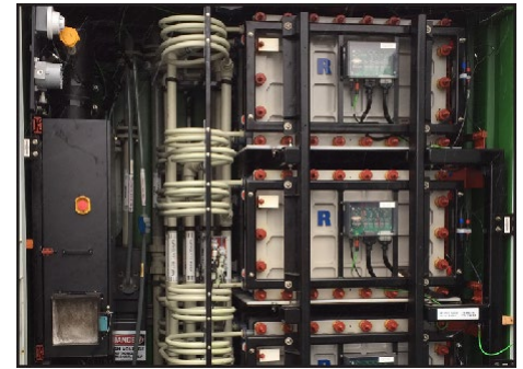
interior of flow battery
