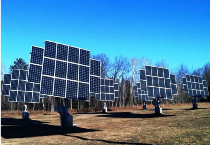
Figure 1: This photovoltaic system consists of 9 dual tracking arrays and is located at the Audubon Center of the Northwoods in Sandstone, MN.
