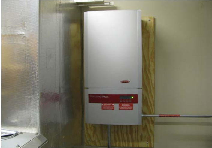
Feronius Converter located in Dining Hall Electrical Room. Last stop for the solar electricity.
