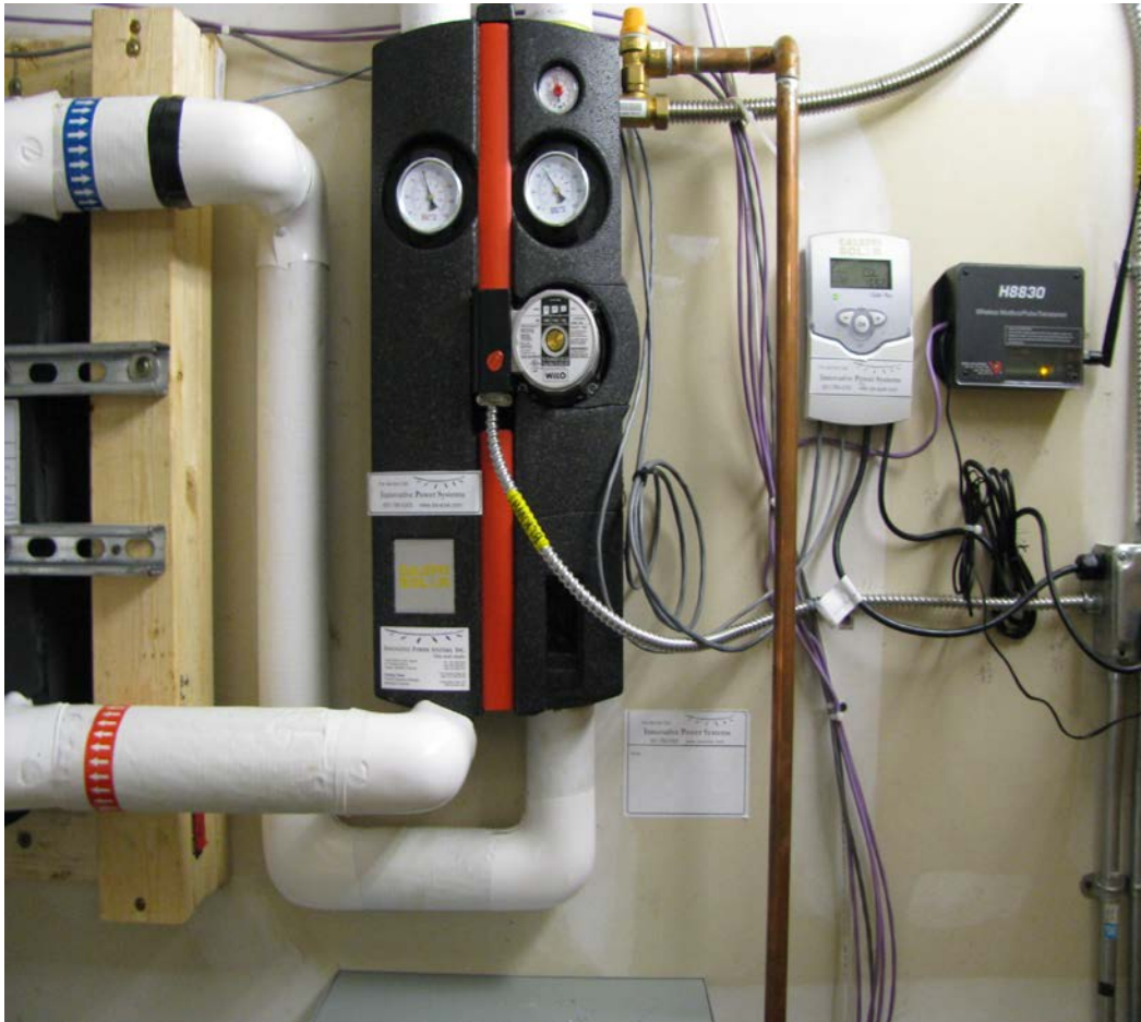
Monitoring equipment at the North Star Lodge for the Solar Hot Water.
