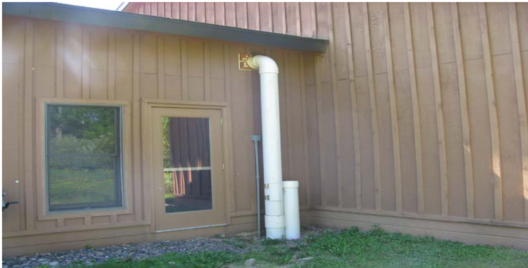
Hot water enters the North Star Lodge, line is protected by PVC pipe.
