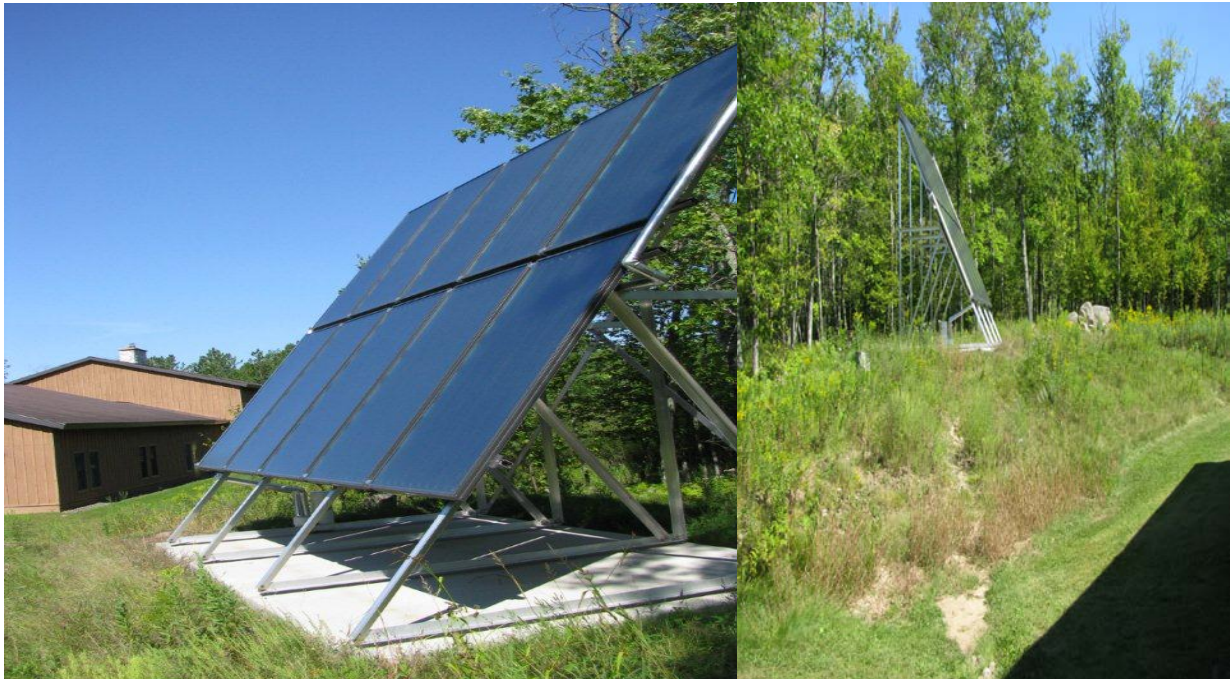
Hot Water Solar Array for the North Star Lodge building at Long Lake Conservation Center. Trenching to the North Star Lodge is still evident in the right hand photo.
