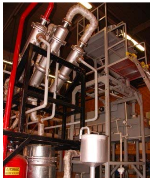
Figure 4. Condenser of the stationary pilot scale microwave pyrolysis system
