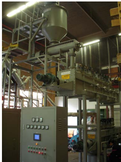
Figure 3. Large pilot microwave assisted pyrolysis system installed at the Center for Biorefining, University of Minnesota.
