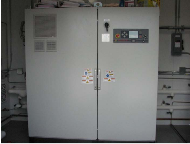
Picture 1. Exterior of the Proton Energy Systems electrolyzer.
