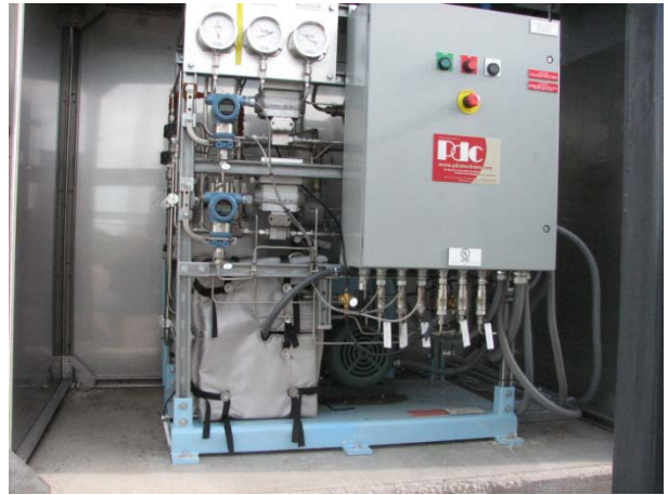
Picture 8. Hydrogen compressor
