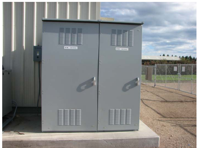
Picture 4. Switchgear to place power on the grid
