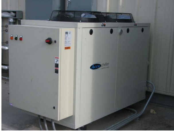
Picture 7. Chiller for cooling electrolyzer and compressor
