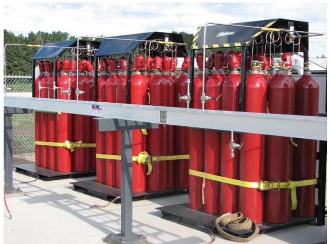
Picture 4. Hydrogen storage tanks
