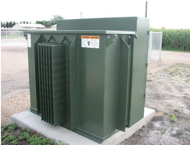
Picture 5. 12.5 kV to 480 volt transformer
