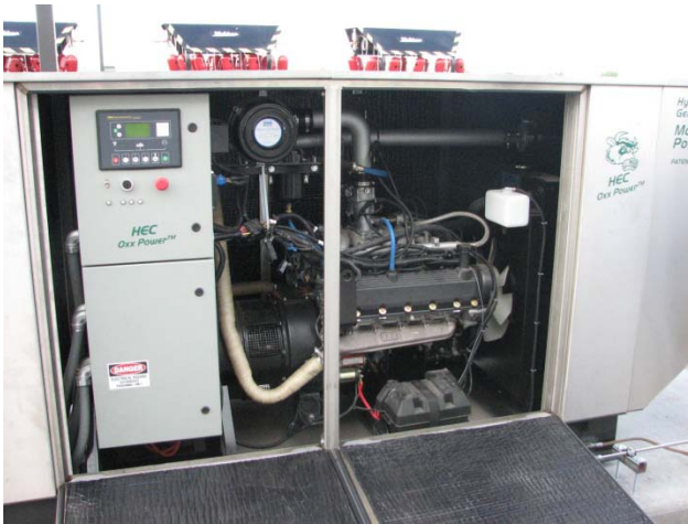
Picture 3. 60 kW hydrogen engine generator set
