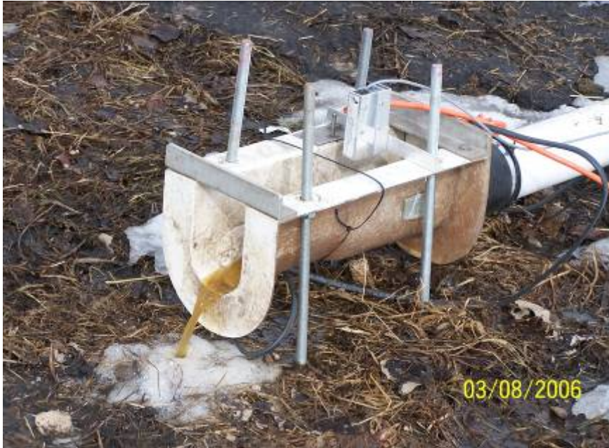
Figure 37: Biofilter discharge flume including flow sensors
