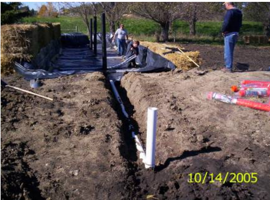
Figure 36: Front view of biofilter with intake pipe (front) and installation of "flow interceptor" H-pipes (back)
